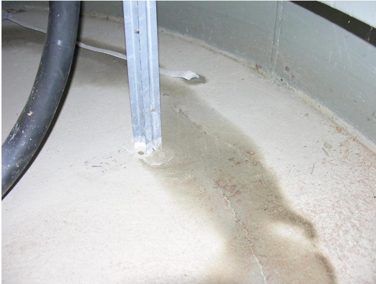
Cracks inside cast down part
