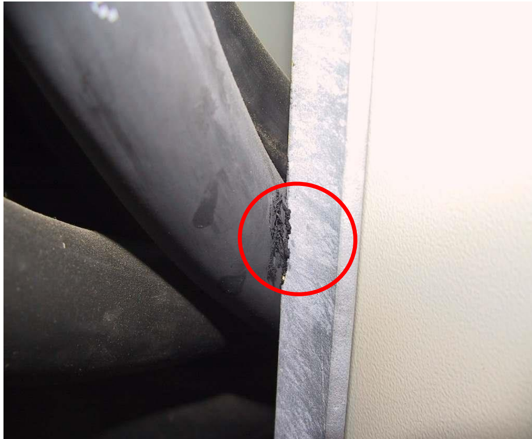
Cables worn on panel frame
