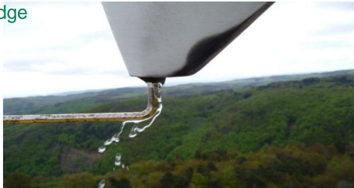
blocked drainage line
